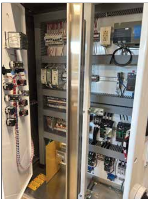
Figure 1 Often the vulnerability isn't in software—it's in the panel where physical access meets controls.
